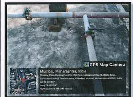
Waste Water In Seepage Tank
